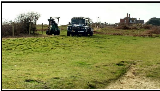
New fencing being installed along the cliff edge on Thorpeness Common, March 2017
