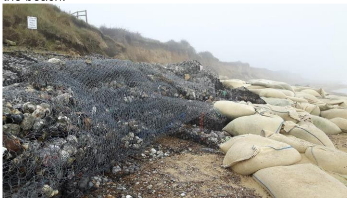
Exposed geobags and damaged gabions on Thorpeness beach
